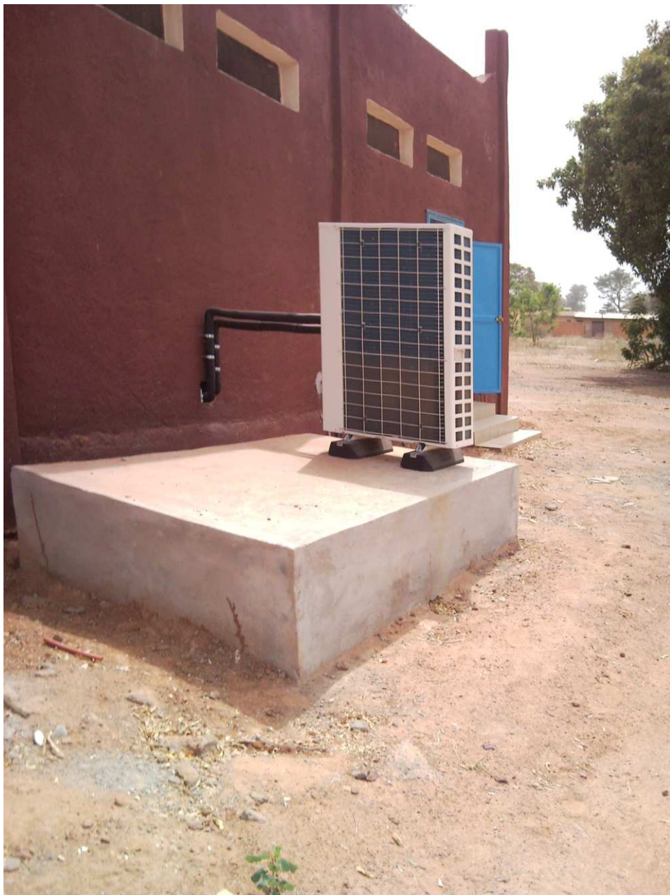
Airconditioning outdoor unit
