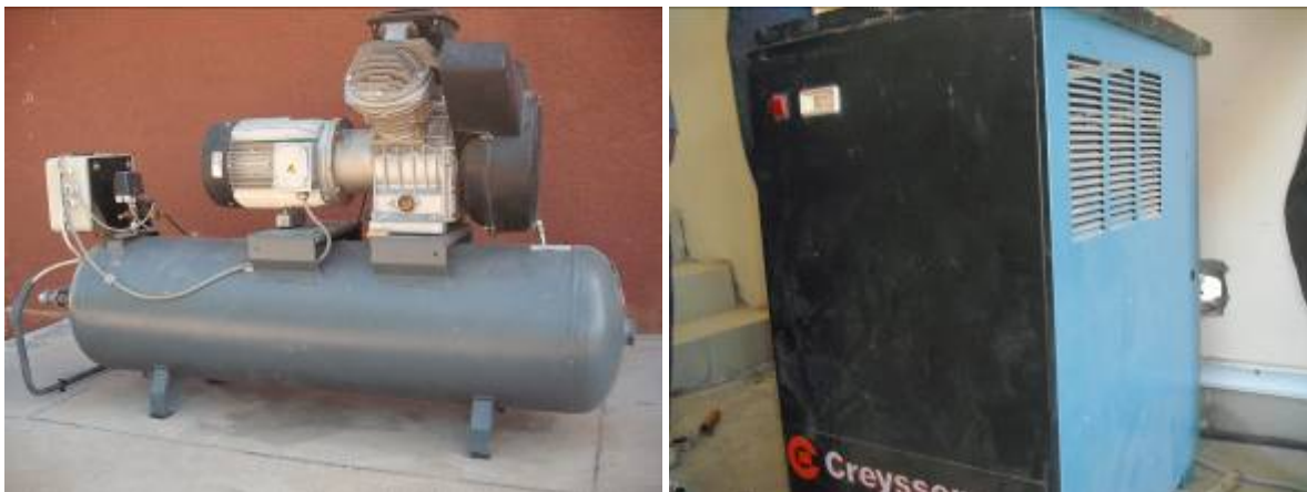
Air compressor and dryer
