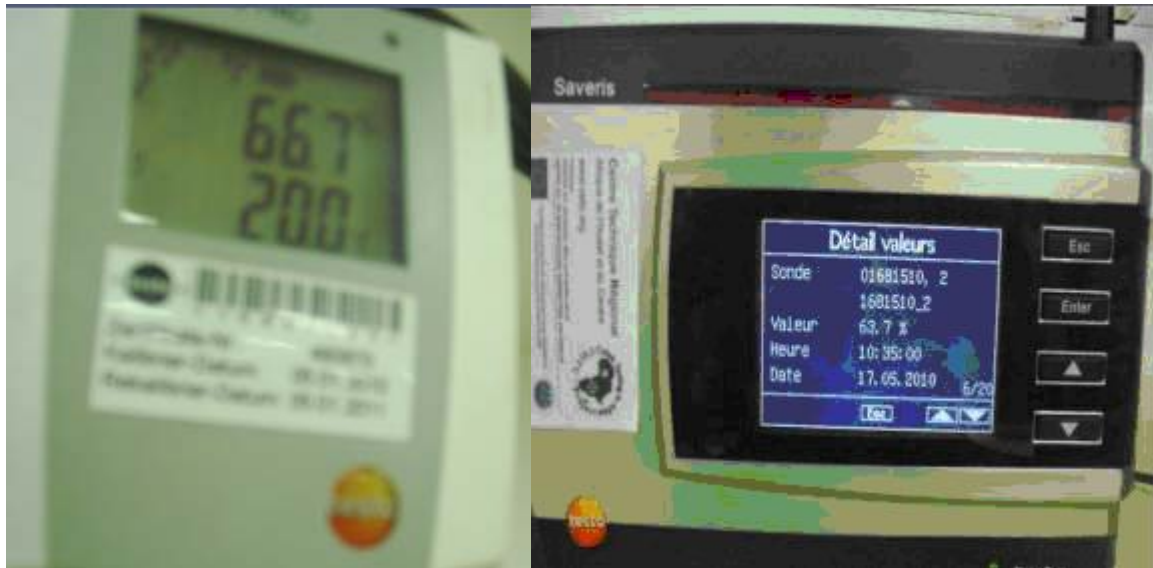
Temperature and humidity recorders, Testo-type base
